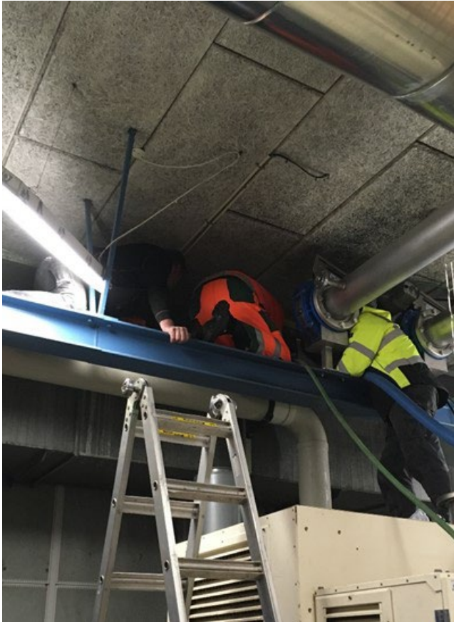
Mounting at Thisted wastewater treatment plant
