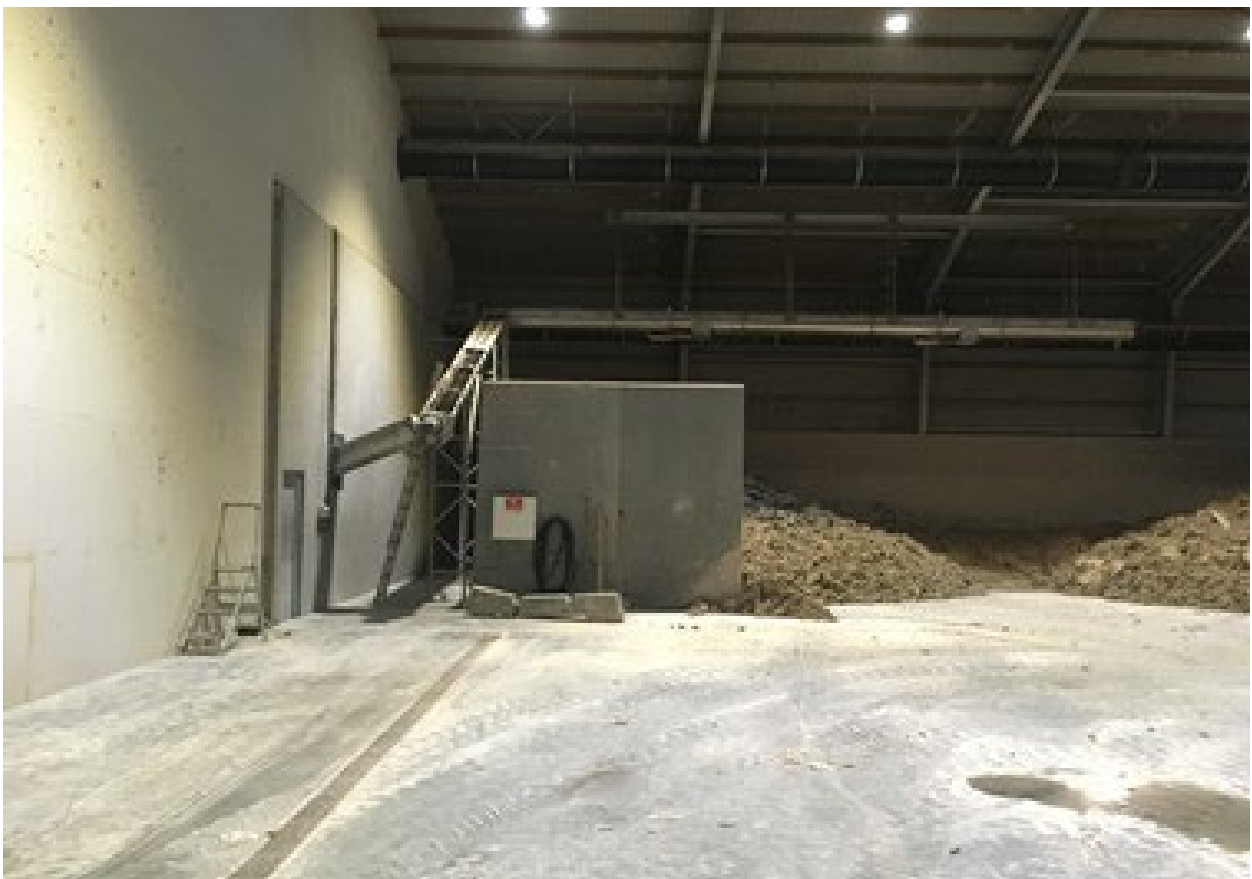
Akselløse transportsnegle i slamlager
