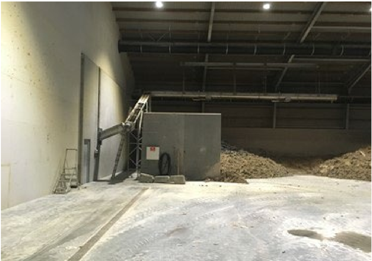
Shaftless transport augers in sludge storage.
