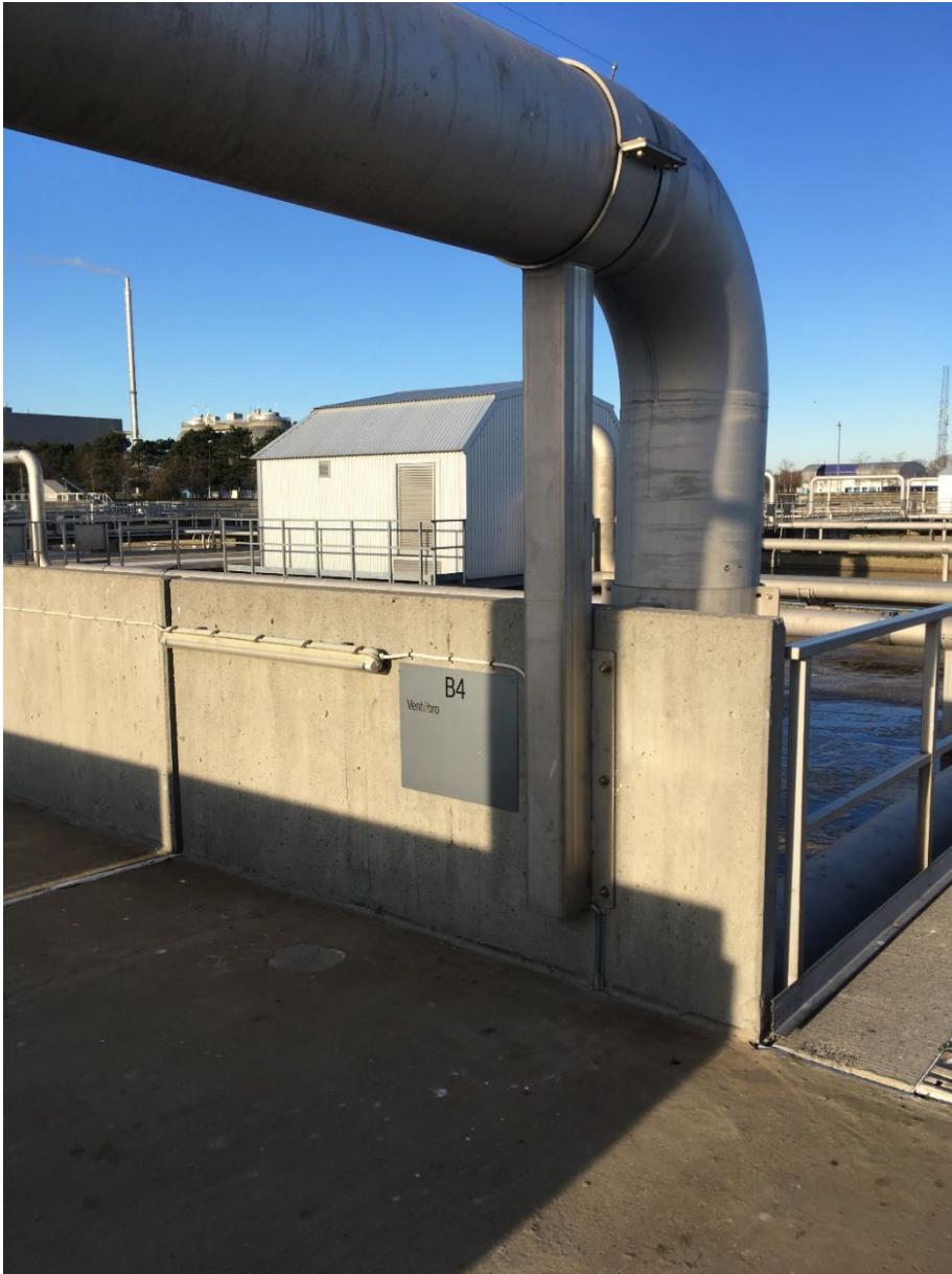
Fan building and piping at footbridge
